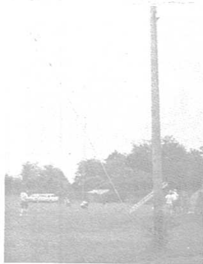
→ UP SHE GOES! NOTE 'GIN' POLE BEING USED TO RAISE 32EL 220 BEAM
